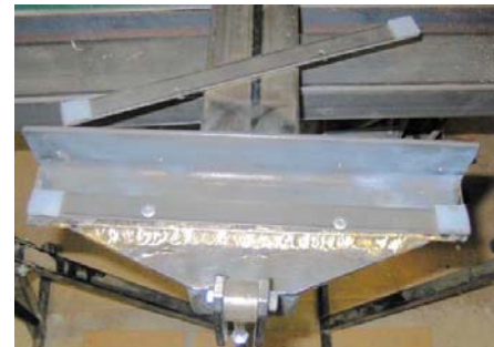
One adjustment plate riveted in place, one resting on the tubing, ready to be clamped and drilled.
